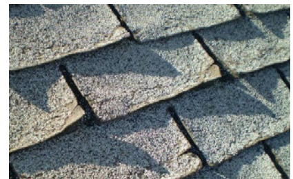
Asphalt roofing will become dry, brittle and misshapen when aged.
