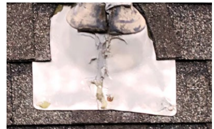
Damaged or aged roof jacks may allow water leaks in your roof.
